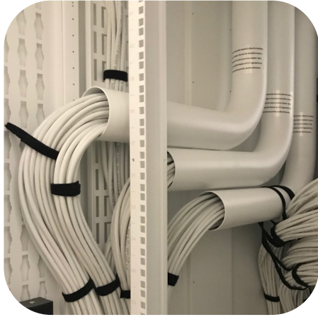
Cable Entry Baffle Pipe
