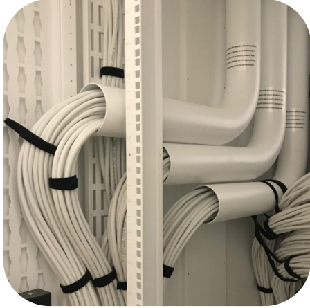
Cable Entry Baffle Pipe
